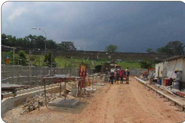
Figure 13: Location where the worker was stationed on the day of the incident.
