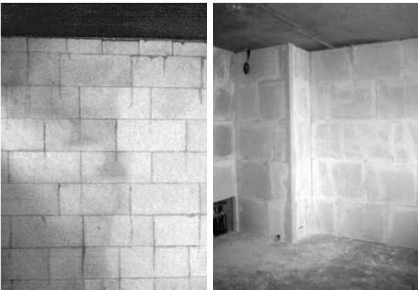
Figure 11 Blocks do not match the storey height
